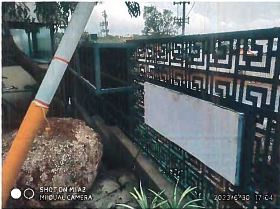
ENTRANCE /SOUTHERN SIDE FENCED WITH BOX SECTION CHANNEL FRAME WITH OPENING GATE.
